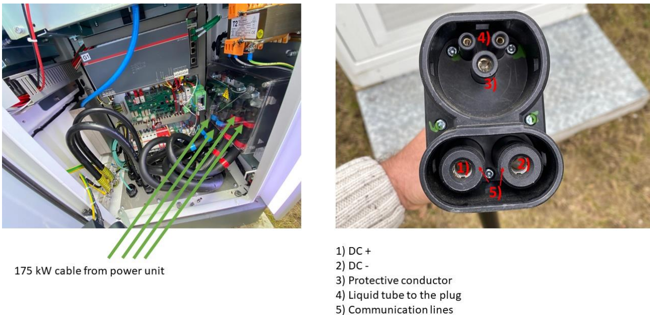
Figure 71. Opened fast charging station (350 kW) and cable for EV charging at Fraunhofer IISB in Erlangen
